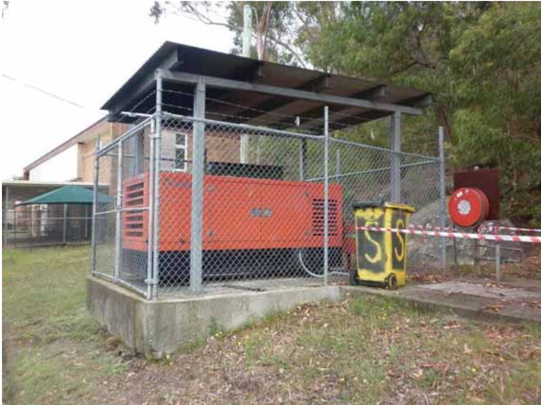
Photograph 5 – Generator on mainland
