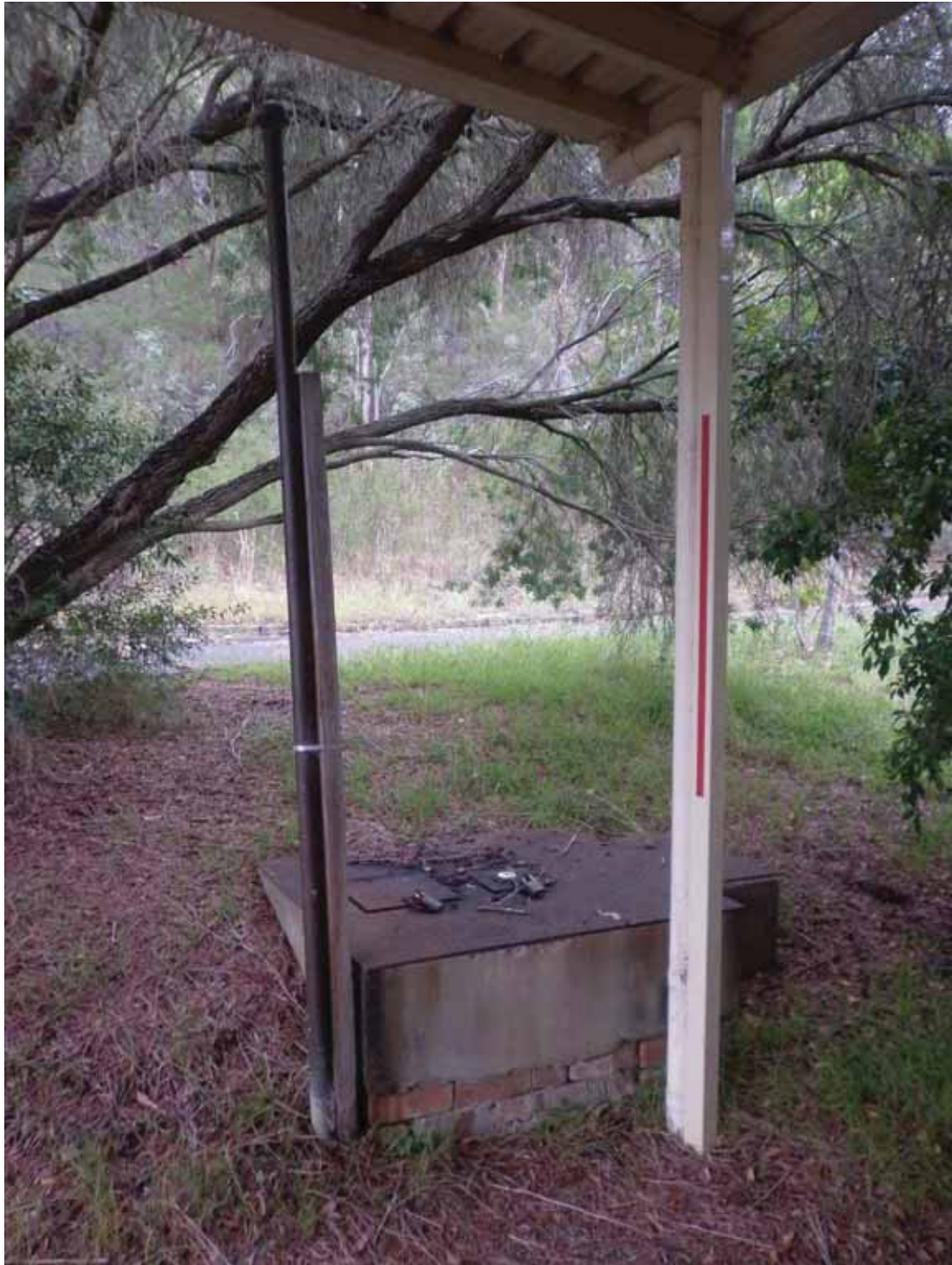
Photograph 4 – Disused UST at rear of former laundry on mainland
