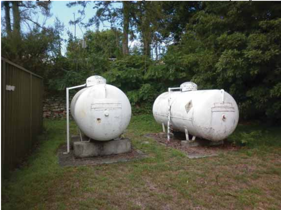
Photograph 10 - LPG Gas tanks on Peat Island
